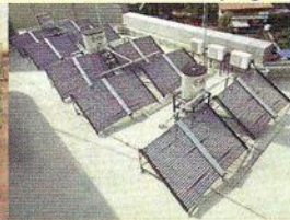
5000 LPD (2 NOS OF 2000 LPD + 1000 LPD)
